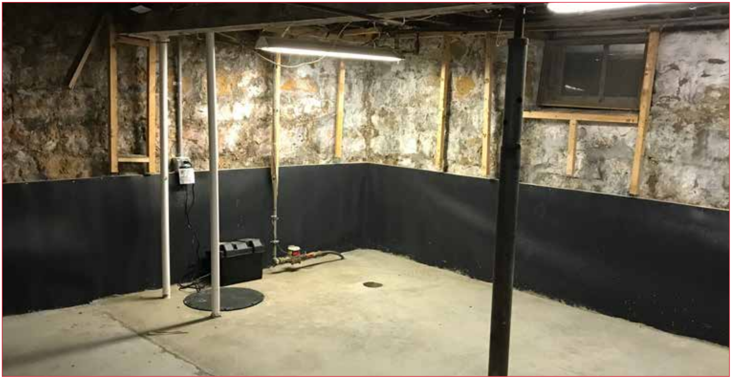
Finished basement project at occupant's home where drainage dimple board, sump pump with battery back up and a humidistat vent fan were installed rendering this space usable for the first time in over a decade.
