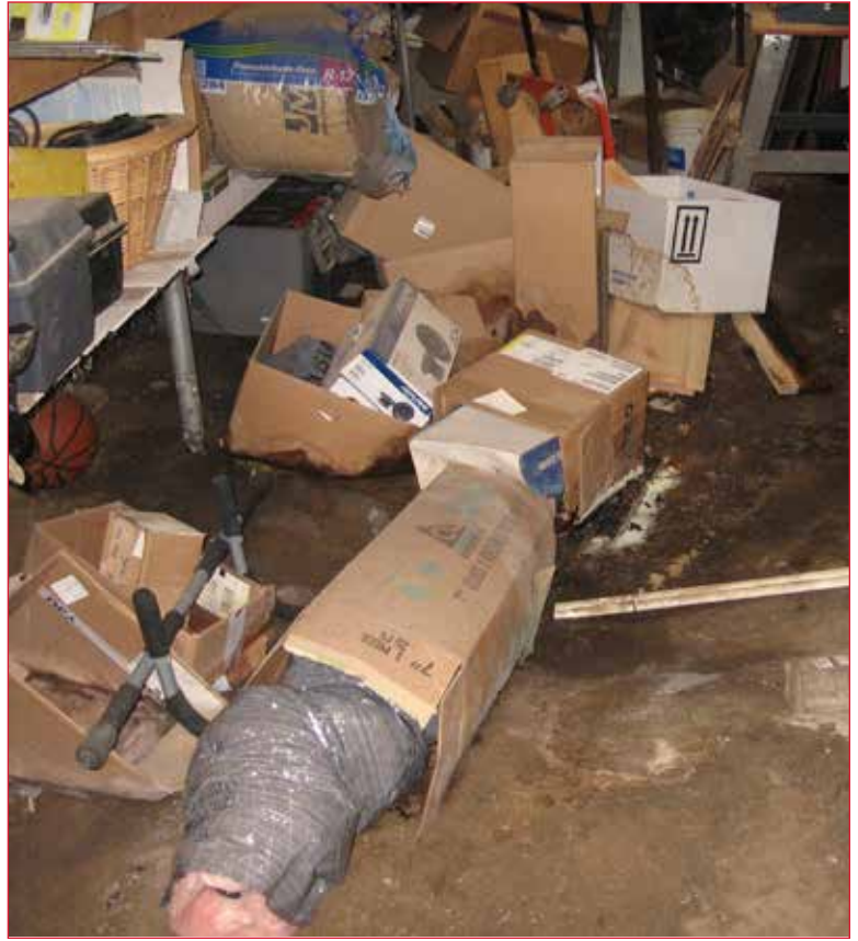
Existing conditions found in the basement of a project after years of water intrusion. Poor Air quality and water wicking materials contributed to asthma triggers for the family living in the home.
